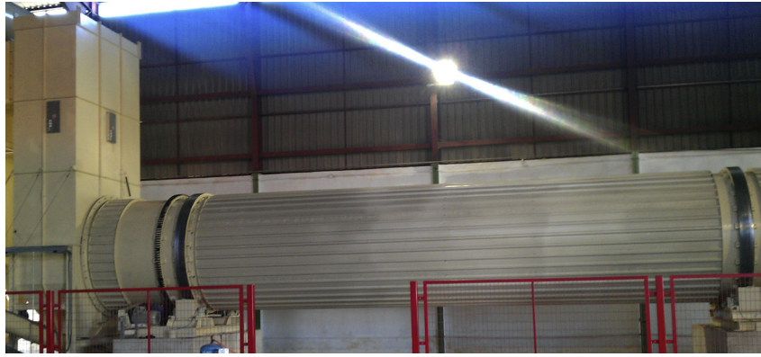
Fig. 1. Trommel in an industrial olive-oil mill waste rotary dryer.
