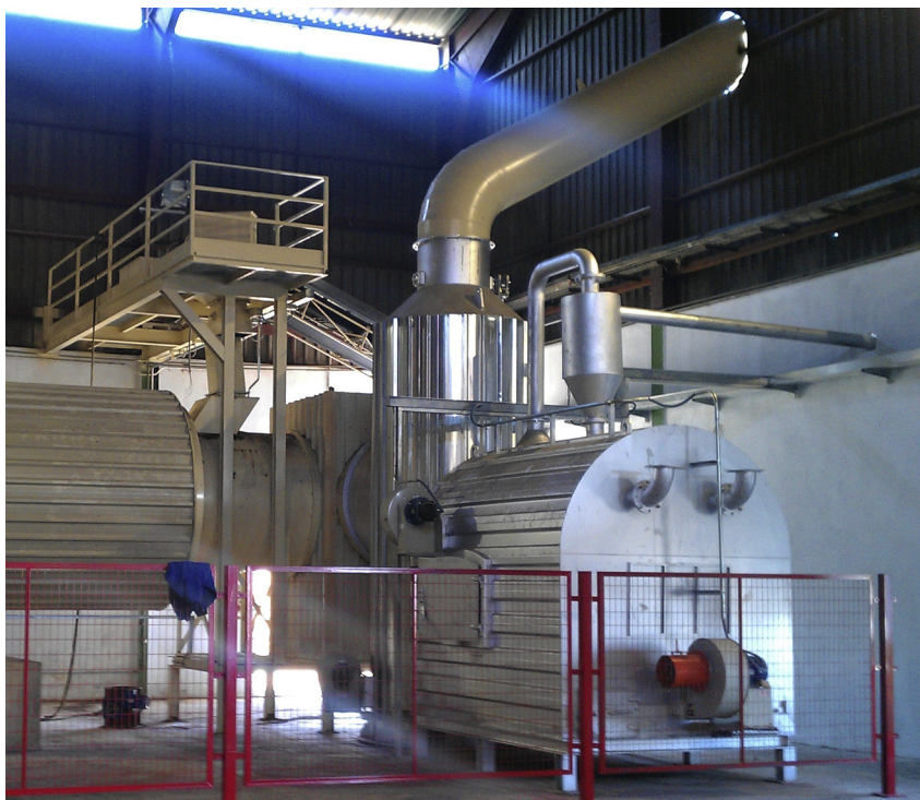
Fig. 4. Furnace in an industrial olive-oil mill waste rotary dryer.
