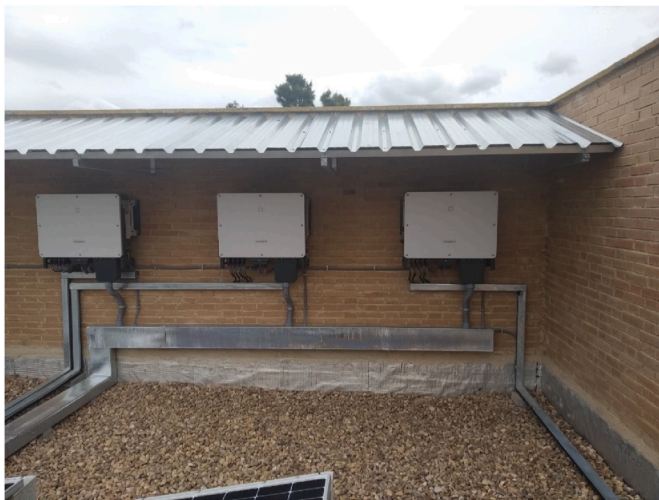
Fig. 4. The three inverters corresponding to Rooftop PV subsystem installed at D3 Building.
