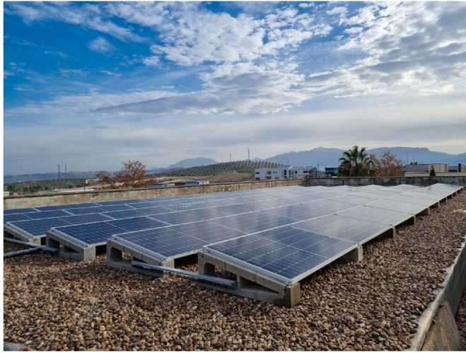
Fig. 3. PV array corresponding to Rooftop PV subsystem at building D3.
