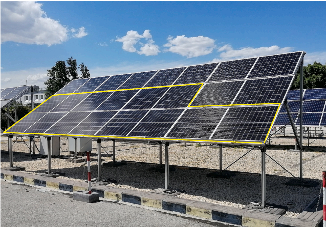
Fig. 1. PV system, front view.
