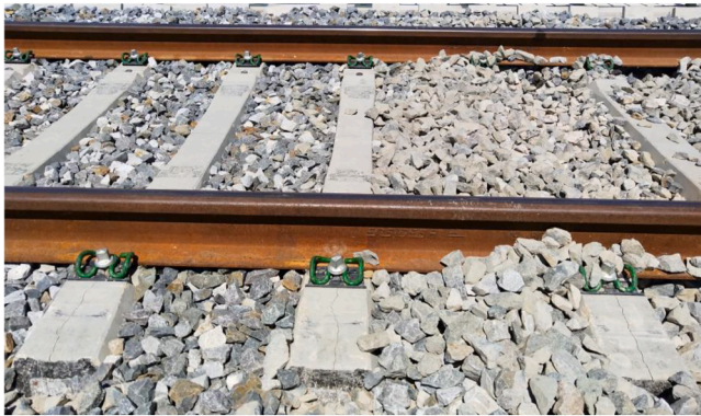
Fig. 1. Cracking in monoblock multipurpose concrete sleepers installed on the railway track.
