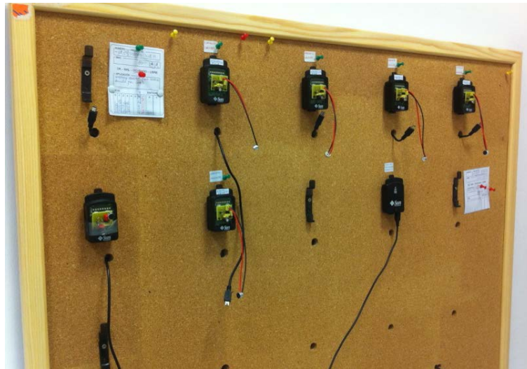
Figura 22. Panel de sensores Sun SPOT del test-bed.
