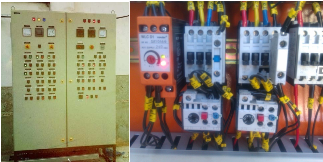
Figure 6.4. Picture of the control panel and specific electric connection.
