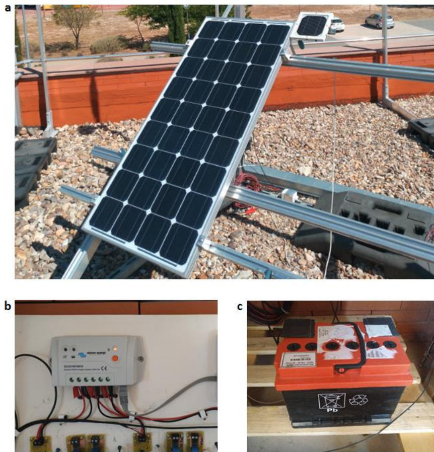
FIGURE 16: SAPV system installation: PV mono-crystalline module (a), charge controller (b) and lead-acid battery (c).
