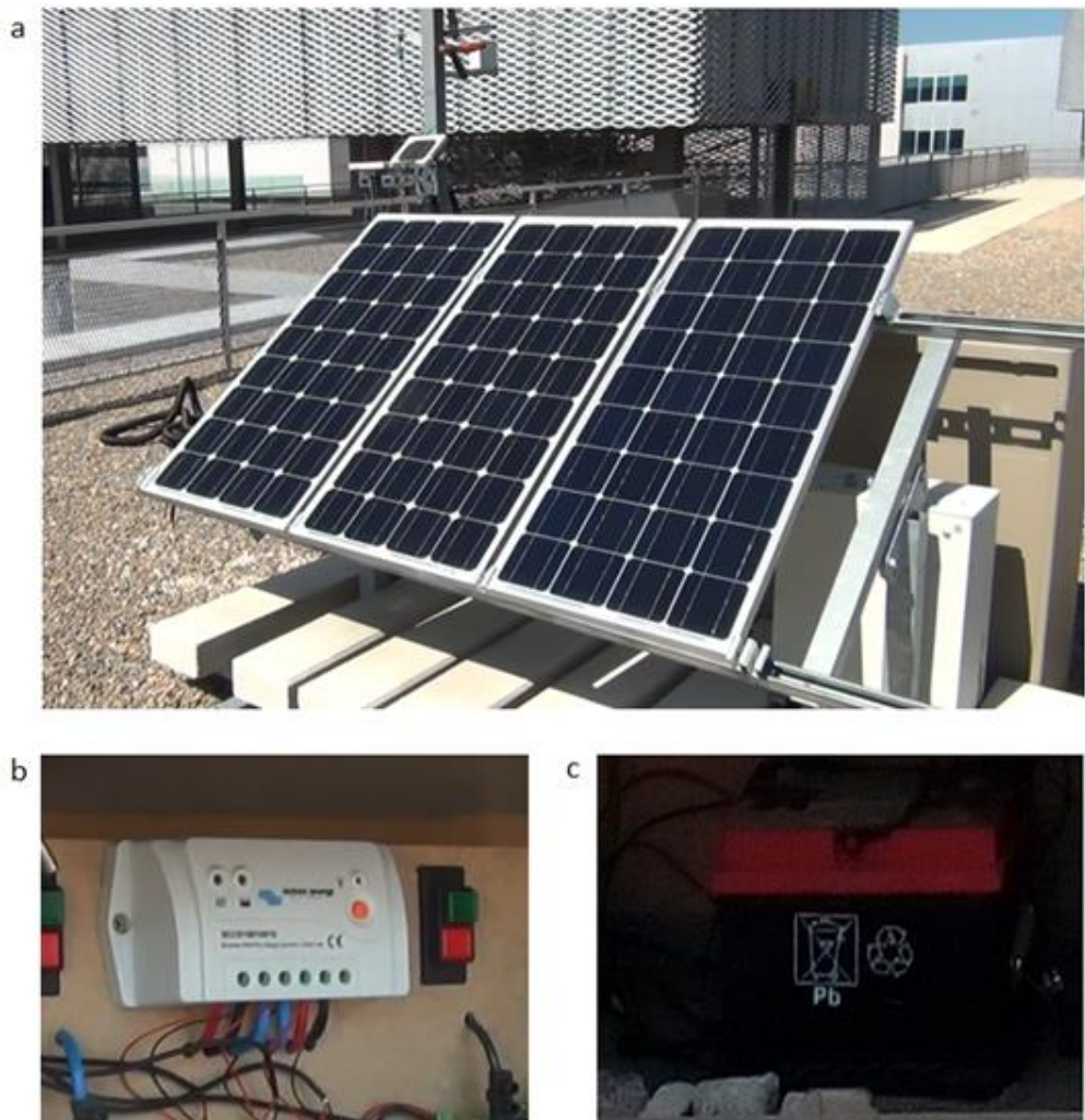
FIGURE 28: SAPV system installed at University of Linares facilities: PV mono-crystalline module (a), charge controller (b) and lead-acid battery (c).
