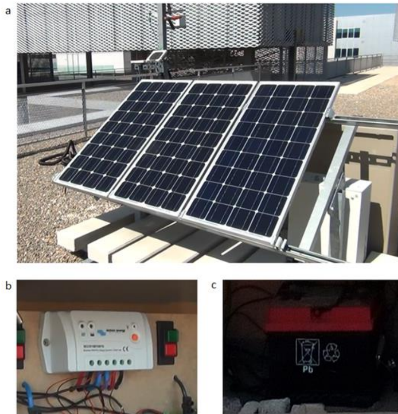
FIGURE 49: SAPV system installation in Jaén: (a) PV mono-crystalline module, (b) Charge controller and (c) lead-acid battery.
