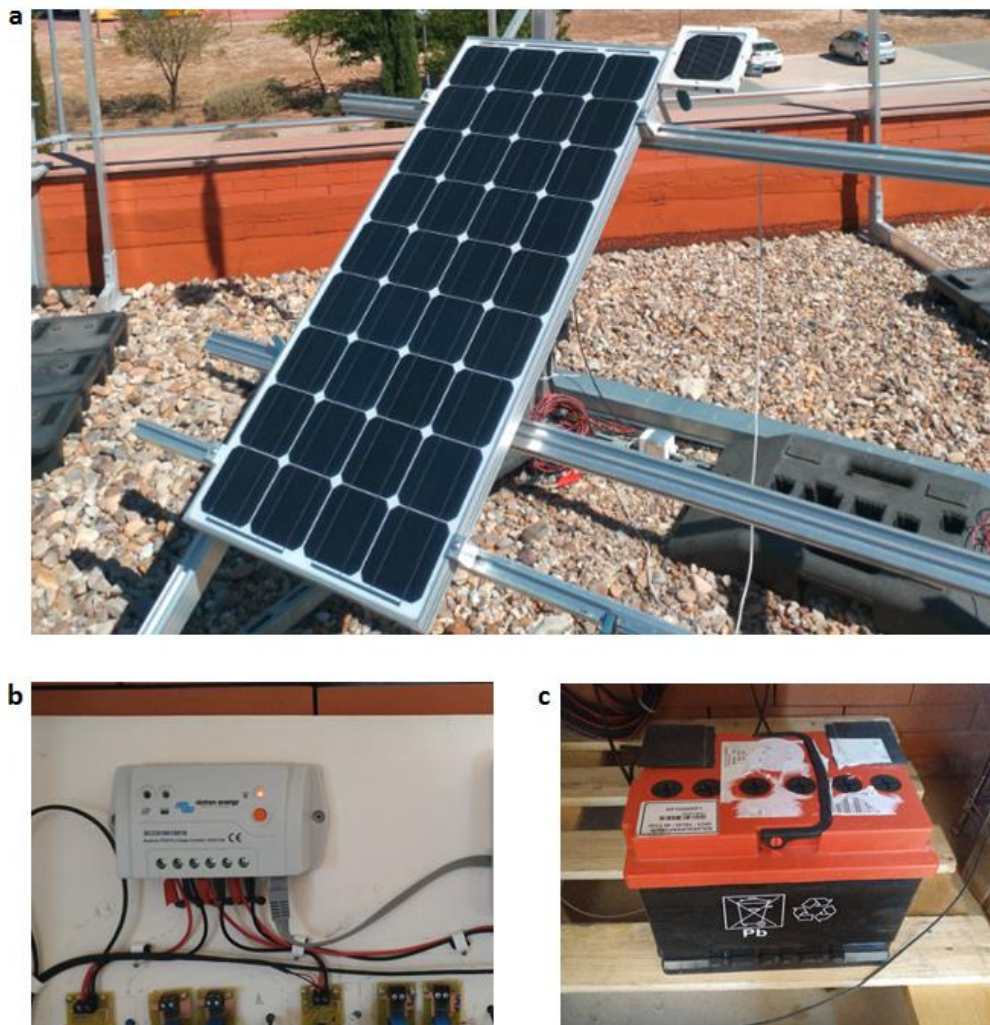
FIGURE 27: SAPV system installed at IMDEA Water Institute facilities: PV mono-crystalline module (a), charge controller (b) and lead-acid battery (c).
