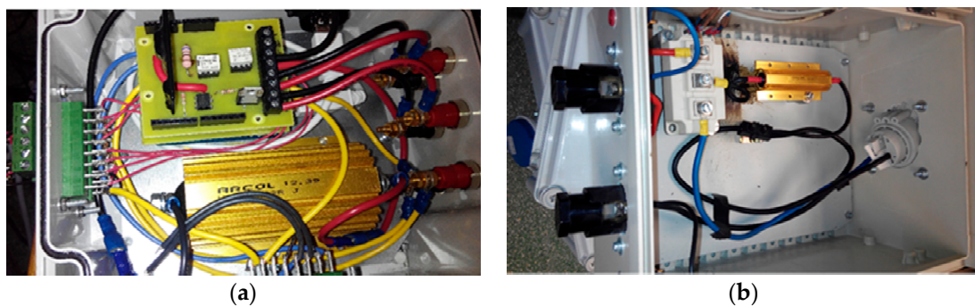
Figure 5. Different designs of the power stage to be used as a function of the size of photovoltaic generator: (a) based on Silicon-Controlled Rectifier (SCR) for charge process, low power electromechanical relays for pre-charge, and solid-state relays for discharge; (b) based on high power Insulated Gate Bipolar Transistors (IGBT) to measure photovoltaic (PV) generators from 20 to 200 kWp.
