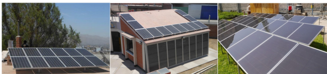
Fig. 1. PV testing facilities (from left to right: Arequipa, Tacna, Lima).
