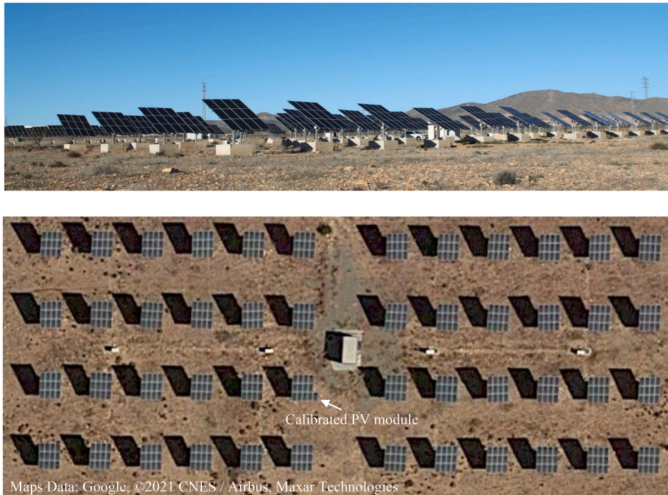
Fig. 3. The 109.44 kW grid-connected PV plant located in Granada, Spain. Top: Photo taken at ground level. Bottom: Satellite photo (Latitude: 37.287, Longitude: -3.057).
