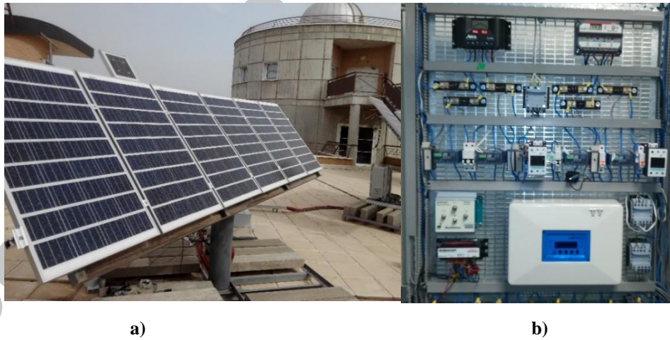
Figure 4 Stand-alone Photovoltaic System (a) PV generator and (b) BCC, sensors and traducers.
