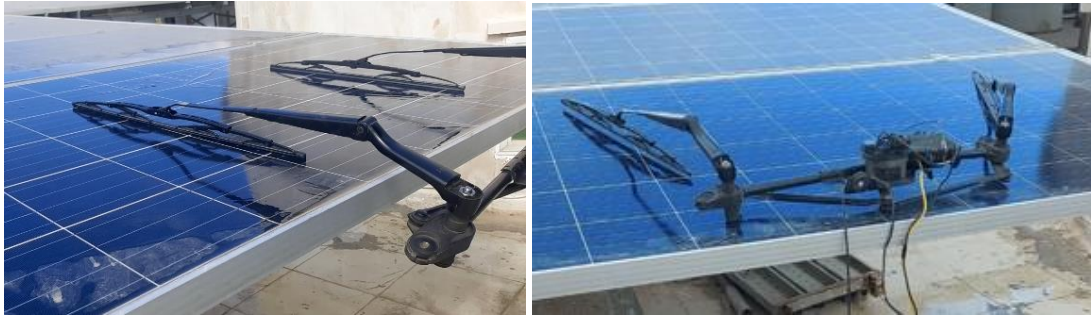
Figure 5 - Cleaning solar panels by car wipers, a pilot project
