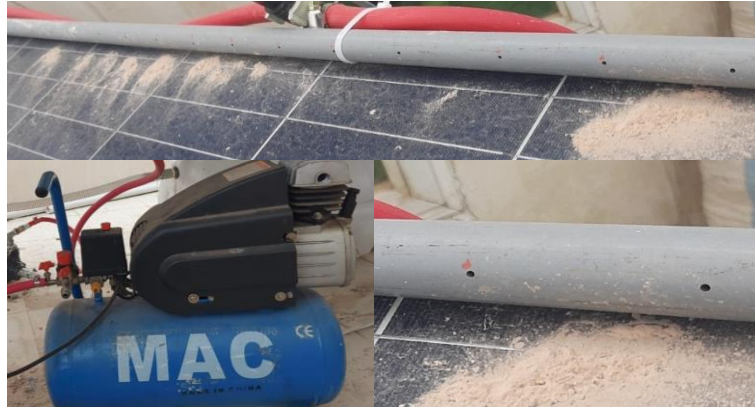
Figure 11 - Air cleaning components utilized in intelligent cleaning system pilot project.
