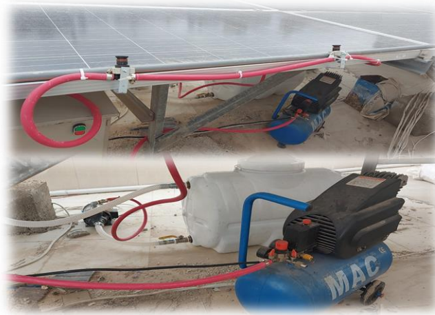
Figure 0010 - Intelligent cleaning system, pilot project
