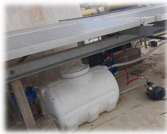
Figure 13 - Water tank used in the project
